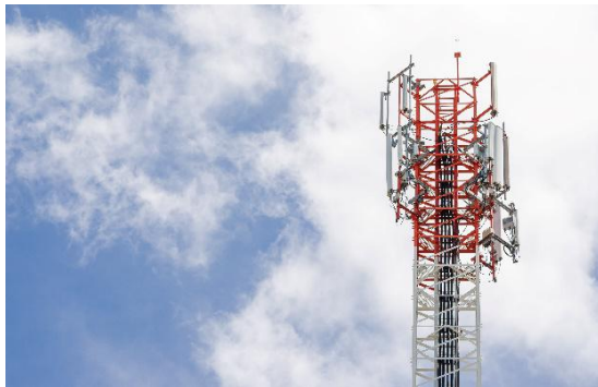
Wireless Infrastructure 无线基础设施
