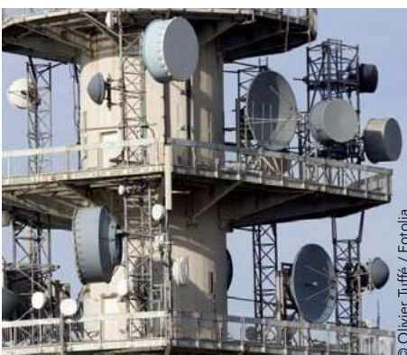
Telecom - Data infrastructure
